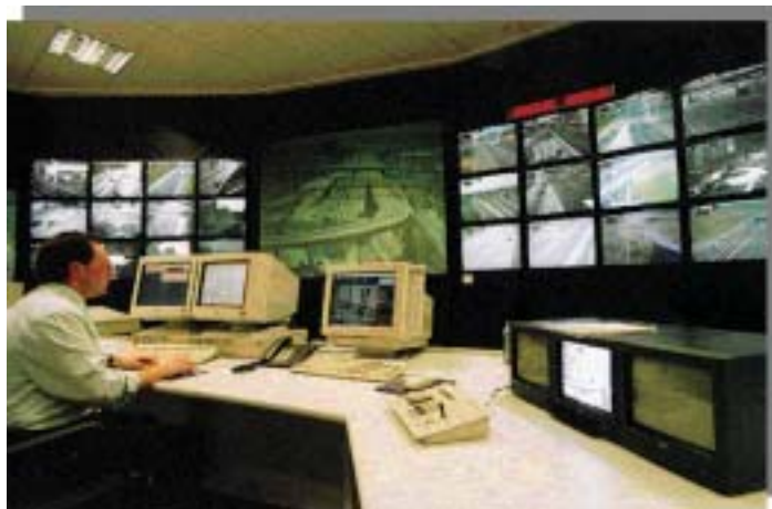
Figure 53. CITRAC and NADICS traffic management center, Glasgow.
